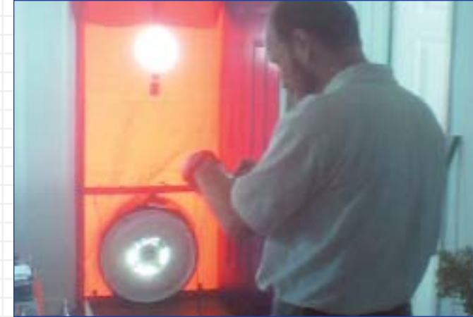
After the Icynene® application, blower door test data confirmed that this home met and exceeded the energy efficient requirements for designation as an EPA Energy Star™ Home.
