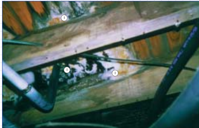
1) Mold problem underneath the floor prior to remediation and installation of Icynene®
