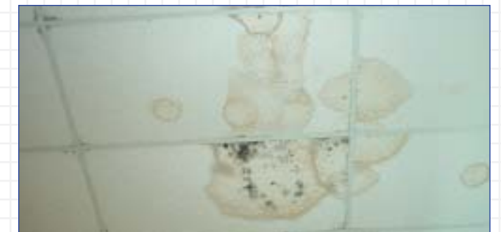
Discolored ceiling tiles were constantly being replaced by Boulineau's who pride themselves on a neat and clean retail environment.
