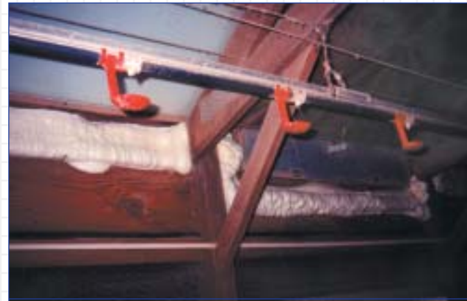
Sealing of the side wall gaps/cracks with Icynene® to prevent air leakage.
